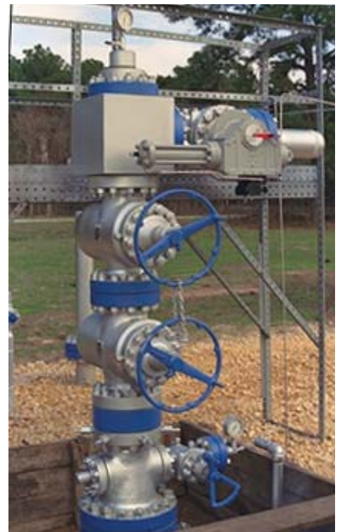
Gas Wellheads and Pipe Lines
