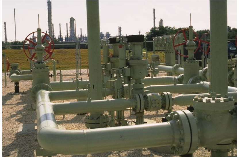
Storage, Metering, and Pressure Reducing Sites
