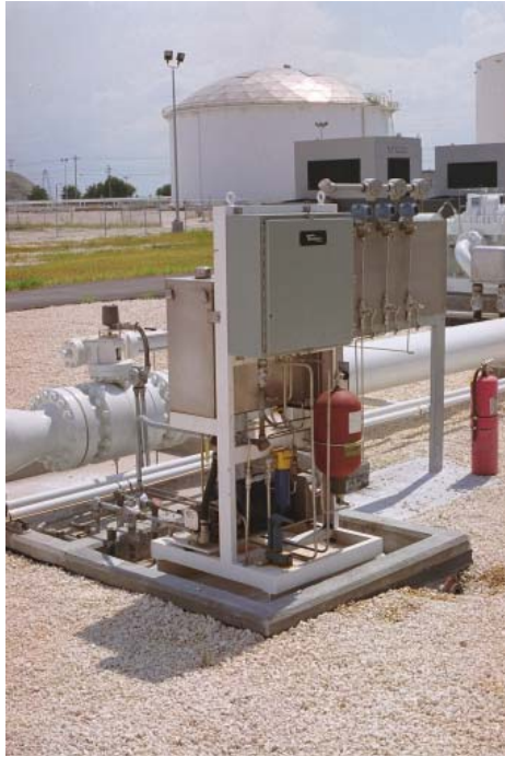
Liquid Pump Stations
